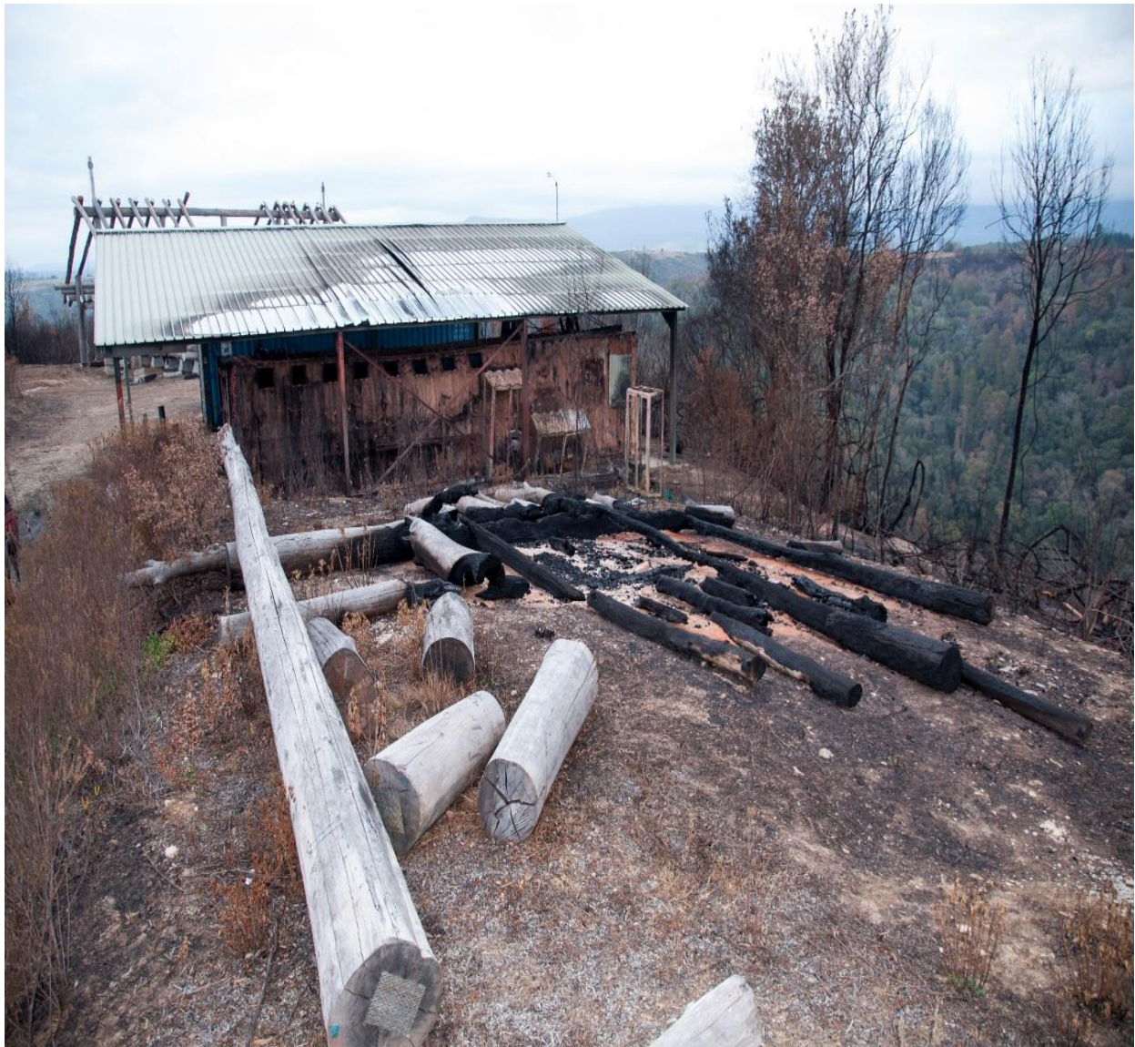
Figure 41: The Eastern side of shed. Note the heat damage to roof. "Noah's Ark" is visible in the background
