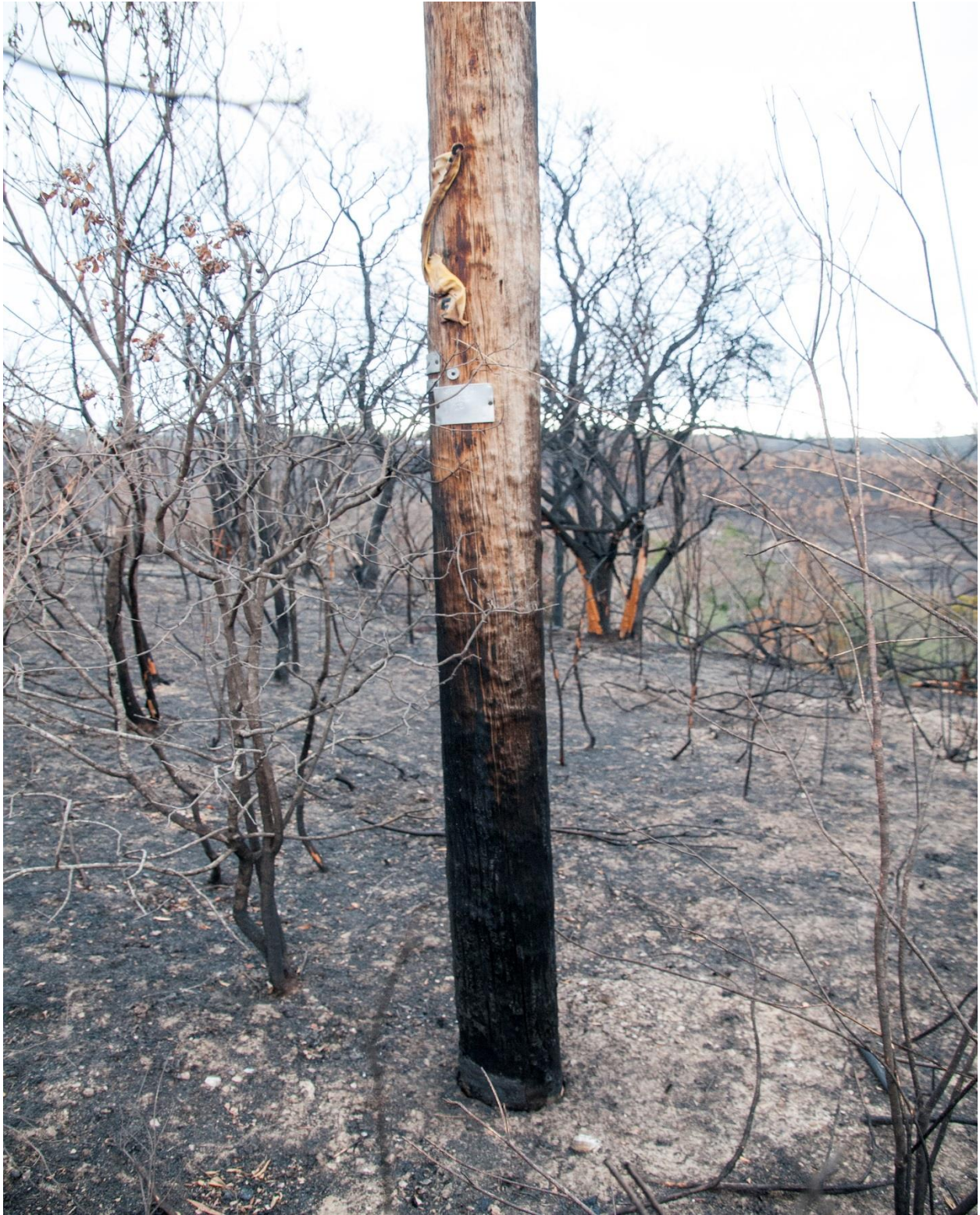
Figure 45: An electricity pole showing fire damage on the Eastern side
