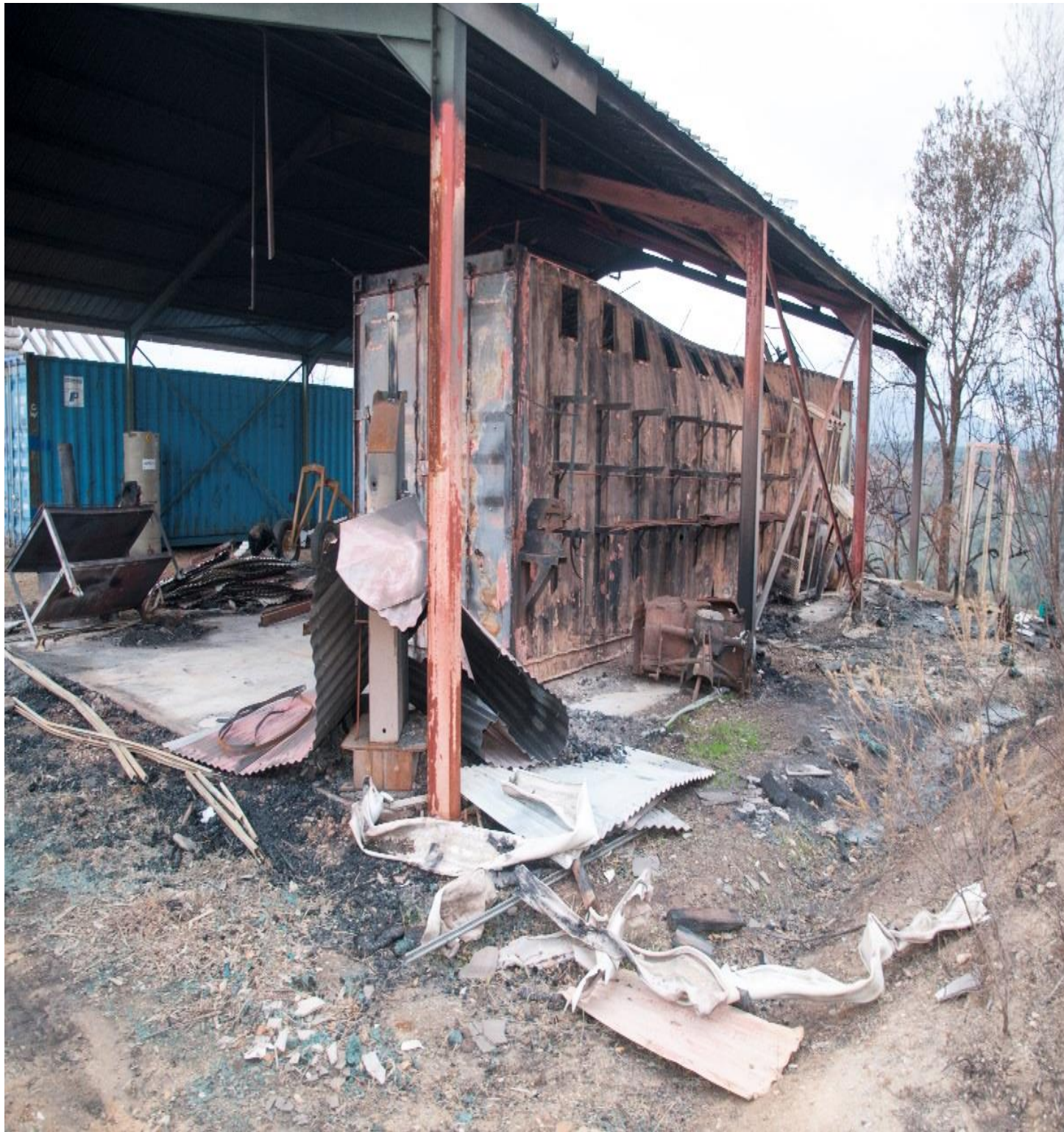
Figure 40: East side of the shed. Note the heat and fire damage on the steel columns and to container.
