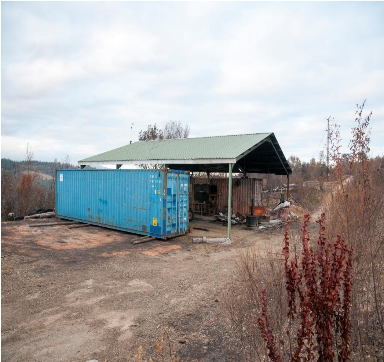
Figure 39: A shed to the East of "Noah's Ark". No burn pattern is visible on Western side of the shed. The container in the photograph moved here after the fire of 07 June 2017. Note that no fire or heat damage on nearest metal column and roof.
