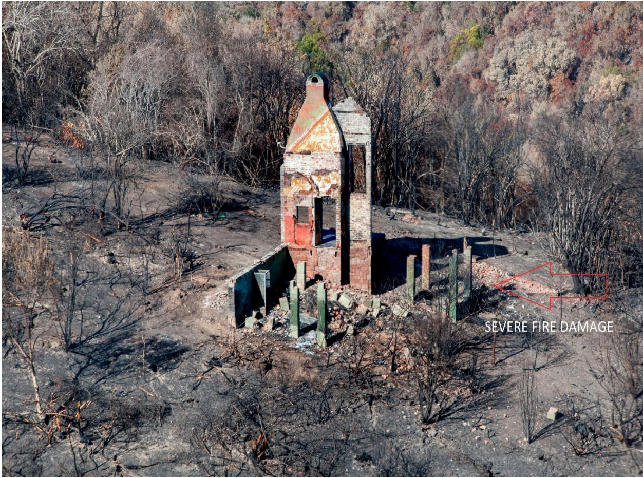
Figure 76: Severe damage from the exposed side with Wind from South-South-Westerly direction.
