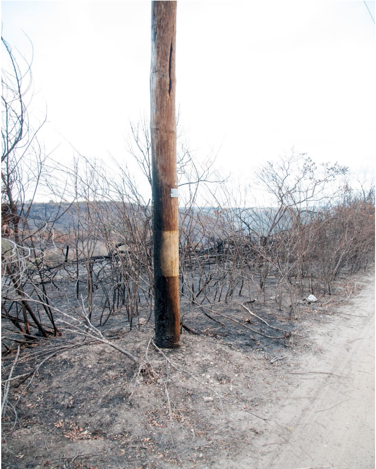
Figure 46: Electricity pole showing severe fire damage on the Eastern side in comparison to opposite Western side
