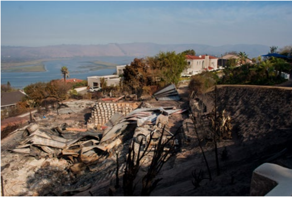
Above: This shows the remains of two wooden homes. These homes were destroyed by embers raining down on vulnerable parts of the homes and/or on vegetation growing up against the home igniting and then causing the home to ignite.
