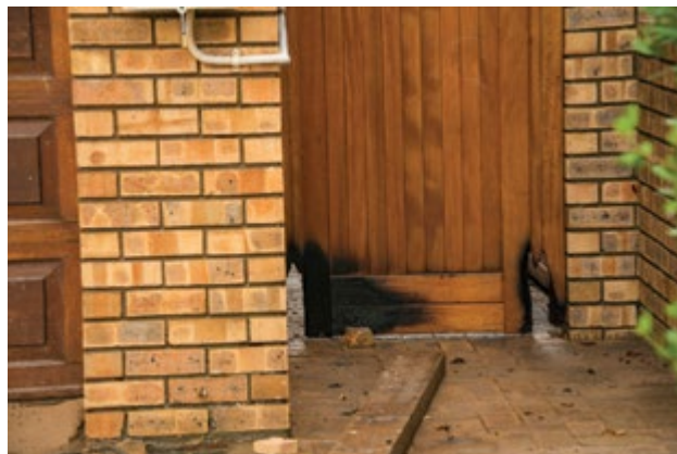
Above: Burned areas of an exterior wooden door clearly show how embers can become lodged and slowly burn the material. Left unnoticed the ignition of this door could have led to the entire home being destroyed.
