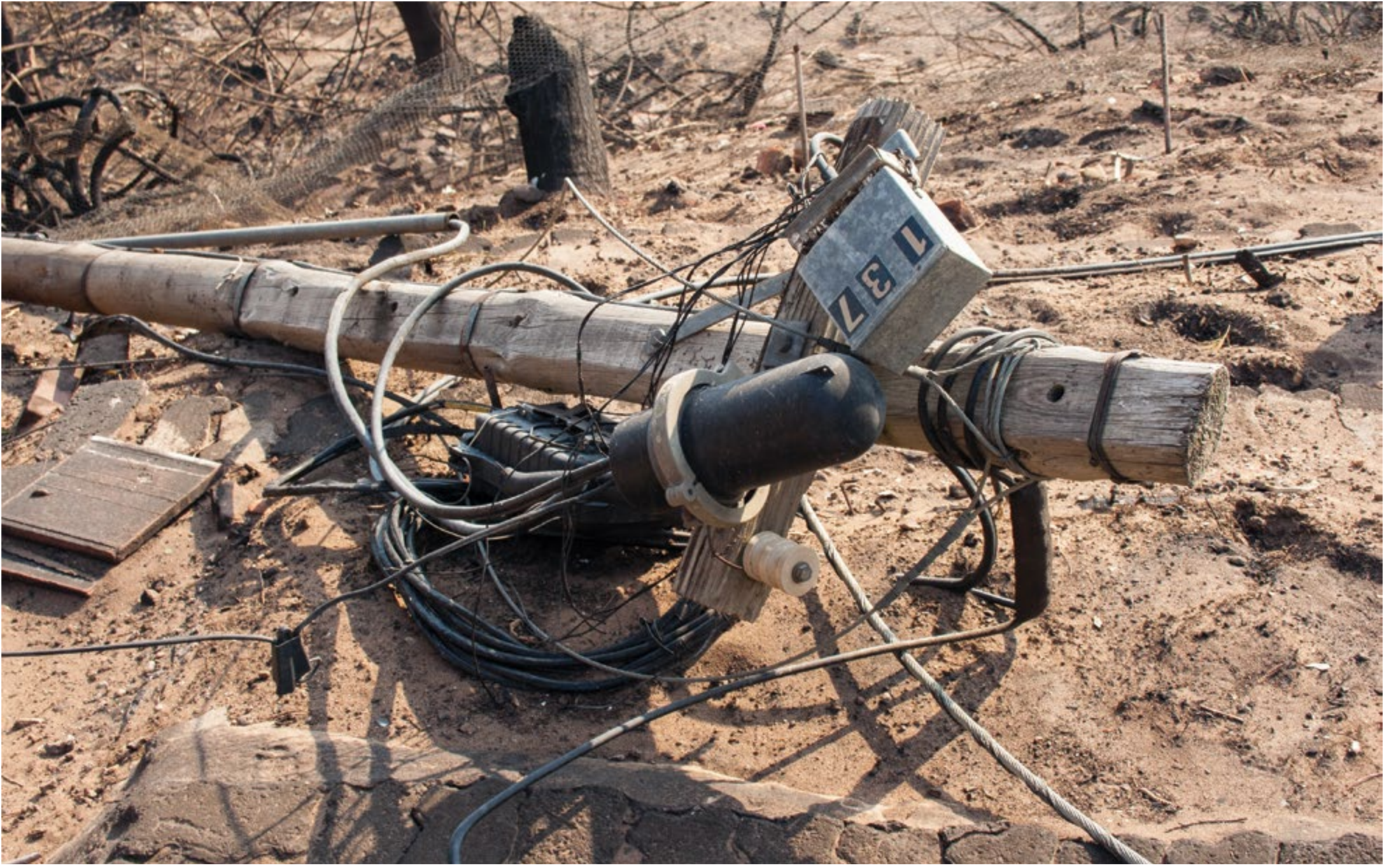
Above: When the land lines went down, the only form of communication was by cell phones which worked at times but were not always reliable. Signal problems due to wildfire-damaged infrastructure as well as battery limitations on the devices were the main challenges.
