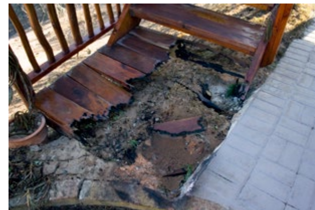
Above: With fine fuel matter and dry grass below the wooden stairs all it took was an ember to ignite the stairs. If there was no one to put out this ignition, it could have resulted in the home connected to the stairs catching alight.
