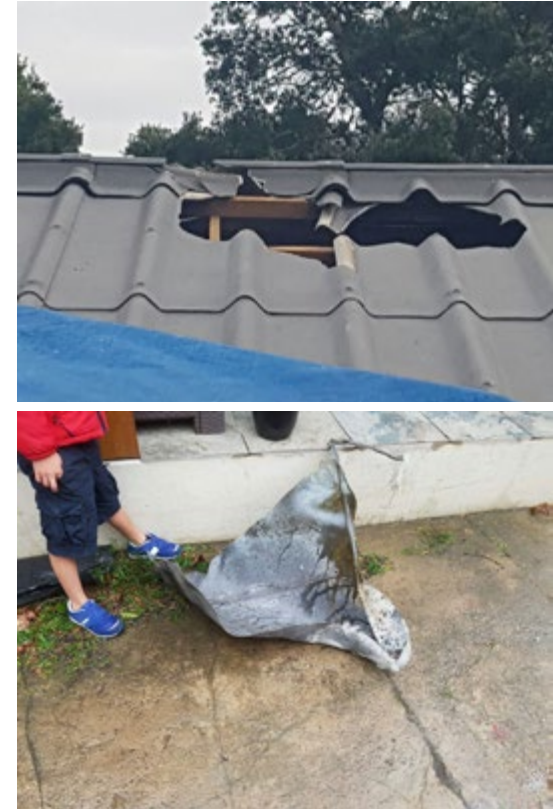
Top and above: Gas bottles that had been left exposed to the radiant heat and flame contact from the wildfires could be heard exploding and some became missiles flying through the air. These could have had lethal consequences. The above image shows the damage inflicted by one gas bottle that exploded, flew through the air and smashed through the roof of a home in Lake Brenton.
