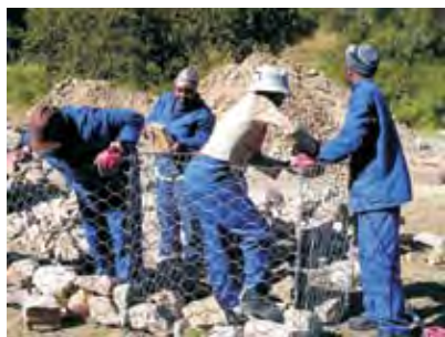
Through the Expanded Public Works Programme, people are being trained and employed to build paths on Table Mountain.
