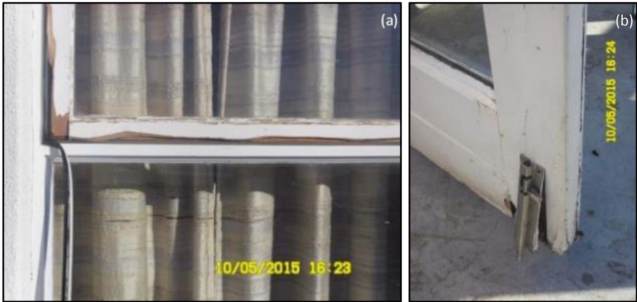
Figure 13: (a) Window damaged and (b) door lock forced open by DG6 in Ocean View.
